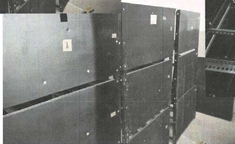
ASSEMBLY OF UPS BATTERY RACK
